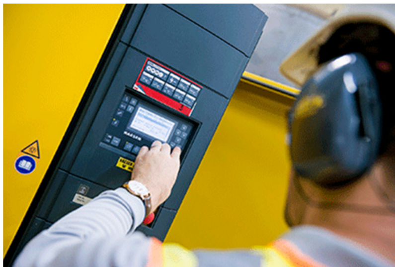
Caption: To reliably and efficiently manage the compressed air system a Sigma Air Manager 4.0 (SAM 4.0) was installed
