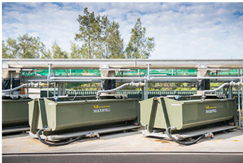
Caption: The new screenings handling area at Malabar WWTP
