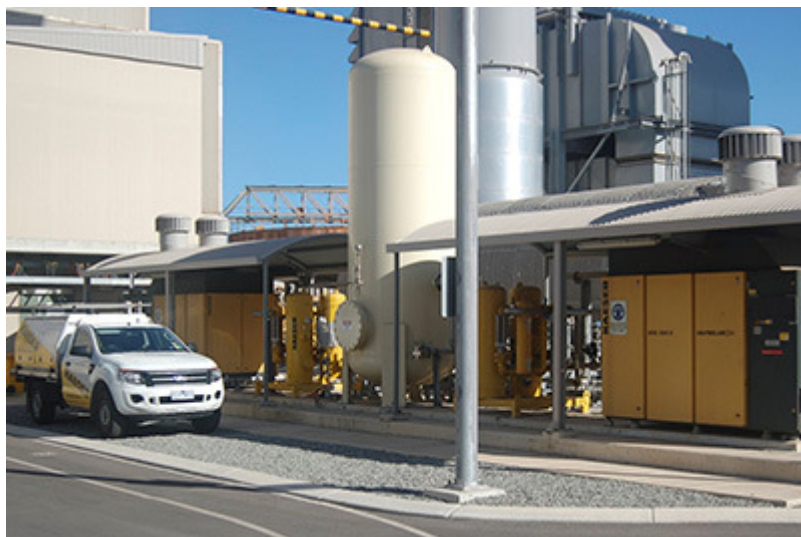
Caption: Four Kaeser DSG-2 series dry-running rotary screw compressors are supplying absolutely clean compressed air to the Kwinana Power Station in WA.
