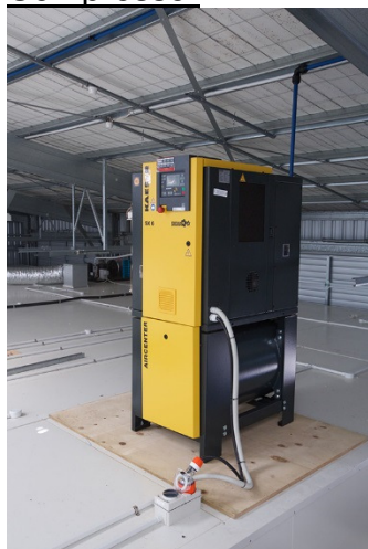
016_Image 2_KAESER compressor at Texas BBQ Foods.jpg
