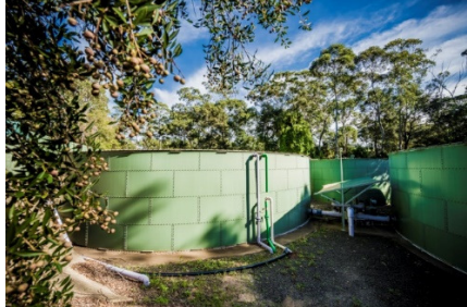
020_Image 8_water recycling plant at PHGC.jpg
