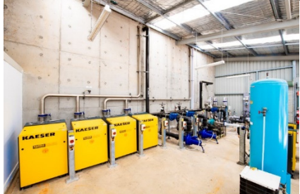
020_Image 3_Kaeser process air at PHGC.jpg
