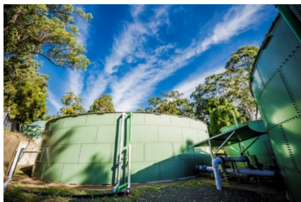
020_Image 7_water recycling plant at PHGC.jpg
