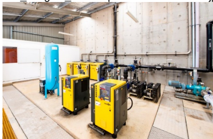
020_Image 4_Kaeser process air at PHGC.jpg
