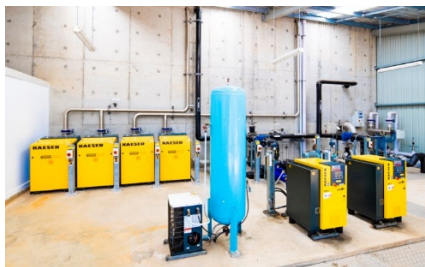
020_Image 2_Kaeser process air at PHGC.jpg
