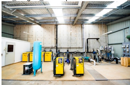
020_Image 5_Kaeser process air at PHGC.jpg
