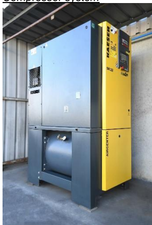
019_Image 1_compressed air at Trucks and Trailers.jpg
