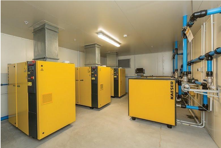
Caption: The complete Kaeser compressed air system that was recently installed at Tasti Foods.
