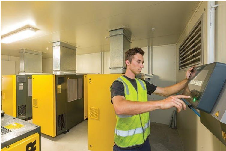
Caption: For maximum efficiency, complete control and connectivity of all components within the compressed air station, a SAM 4.0 master controller was installed.
