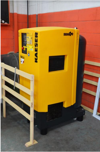
Caption: The Kaeser.SXC 8 all-in-one compressed air supply system at Fisher West Auckland.
