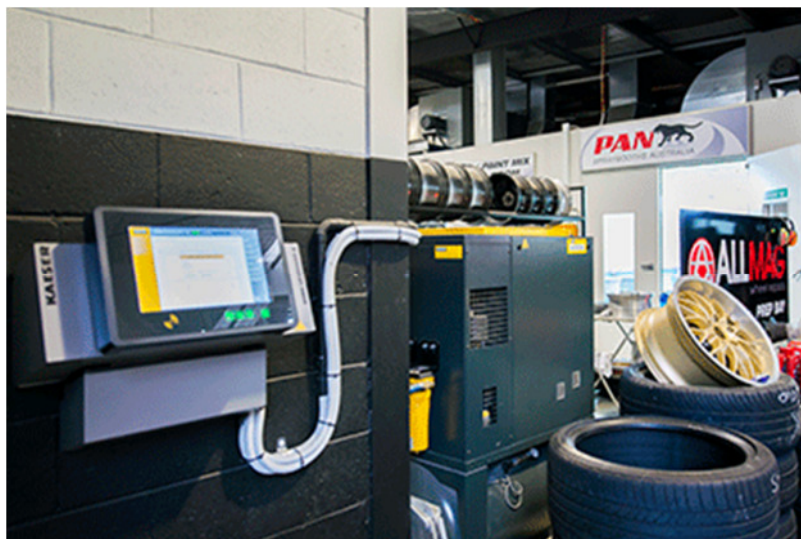
Caption: For optimum efficiency and connectivity, All Mag chose to install a Sigma Air Manager (SAM)
