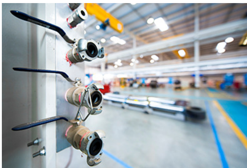
Caption: With seven manifold outlets installed at different points throughout the facility, compressed air is highly accessible when and where required.
