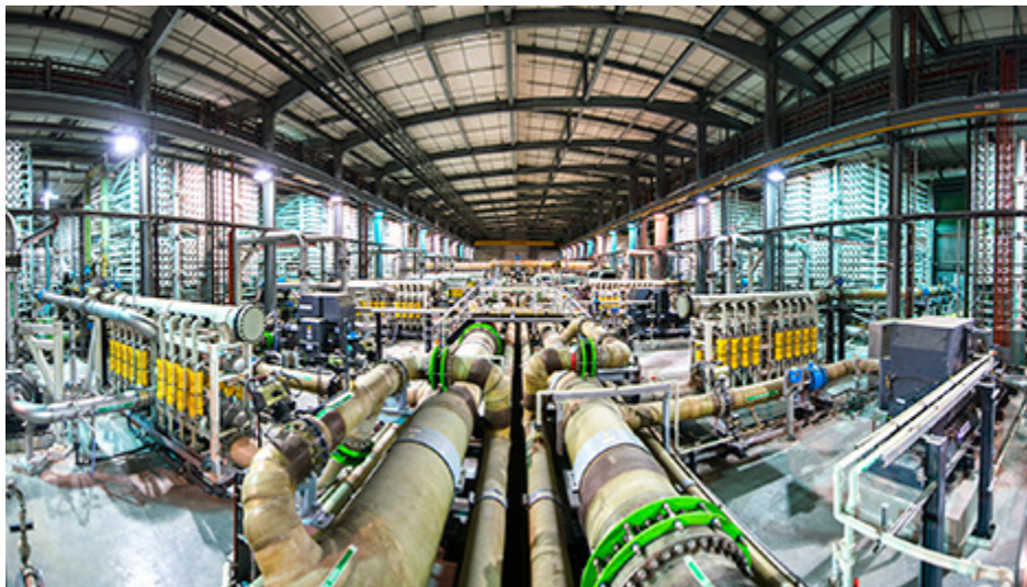
Caption: One of the main requirements for compressed air on the VDP is to actuate a number of the 17,000 plus automated valves
