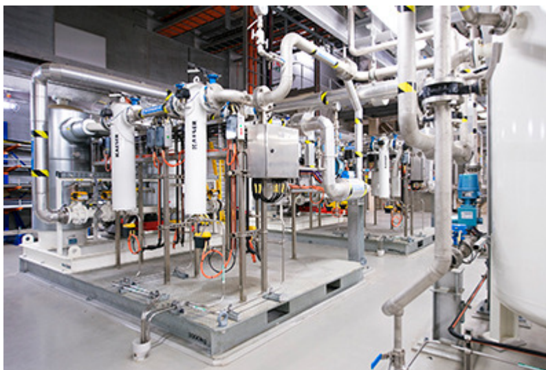
Caption: The VDP utilises 4 air receivers and 4 instrument air treatment skids which include pre- and post- duplex filter sets as well as a desiccant dryer
