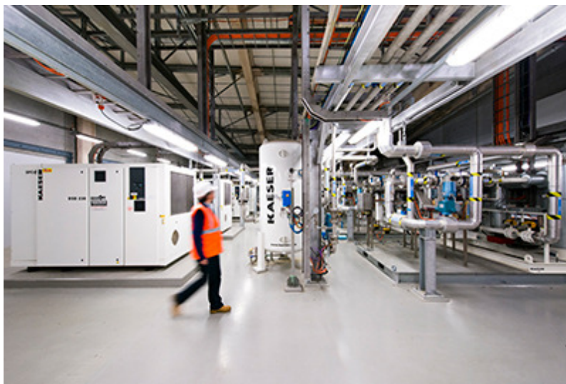
Caption: The VDP utilises 4 Kaeser DSD 238 SFC series frequency controlled rotary screw compressors
