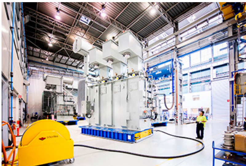
Caption: Powered by the Kaeser compressors, the air skates at WTC can lift up to 300 tonnes of weight and are responsible for moving the transformers into the testing bay.
