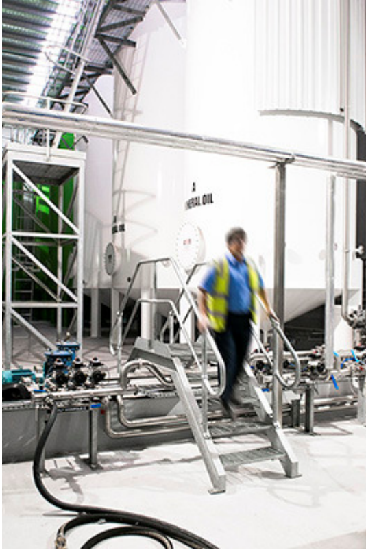
Caption: Compressed air is used to power a number of operations at WTC including powering the pneumatic controls on the oiling system.
