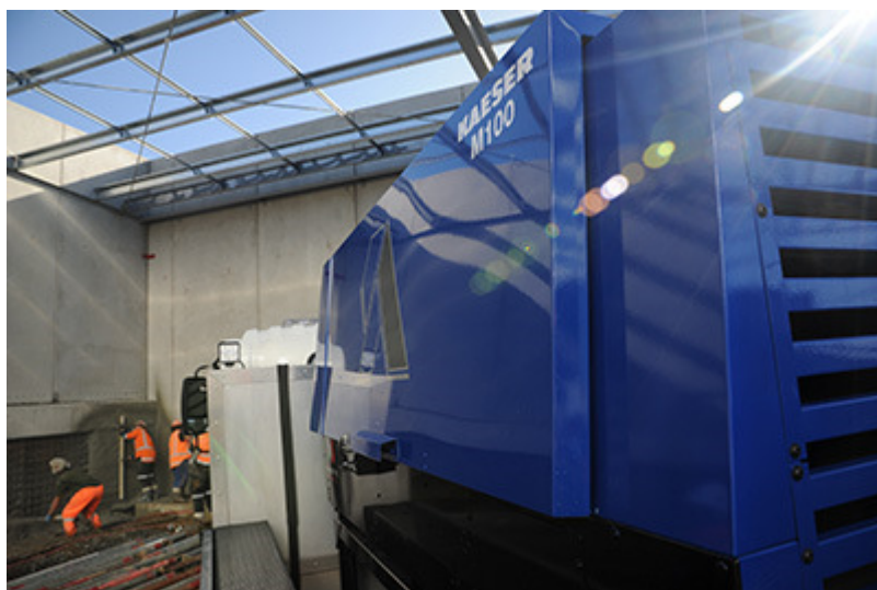
Caption: Shotcrete Auckland recently invested in a Kaeser Mobilair 100 portable compressor
