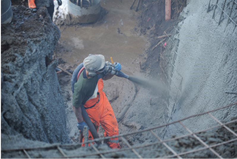
Caption: The cement mixture is pumped through a hose and then pneumatically sprayed onto a surface
