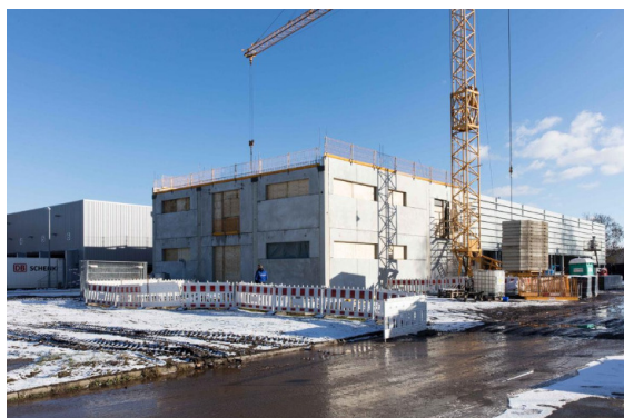
Topping out ceremony at Kaeser: Refrigeration dryers will be built in the new hall soon.
