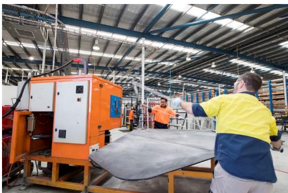
015_Image 6_compressed air application at Prowler Proof.jpg
