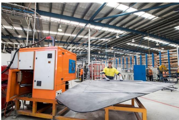
015_Image 7_compressed air application at Prowler Proof.jpg
