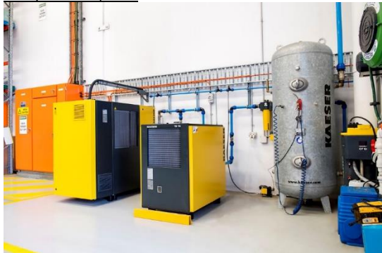
015_Image 1_compressed air at Prowler Proof.jpg
