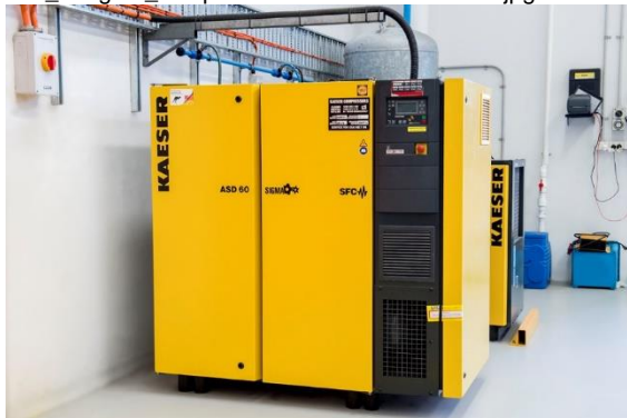
015_Image 2_compressed air at Prowler Proof.jpg
